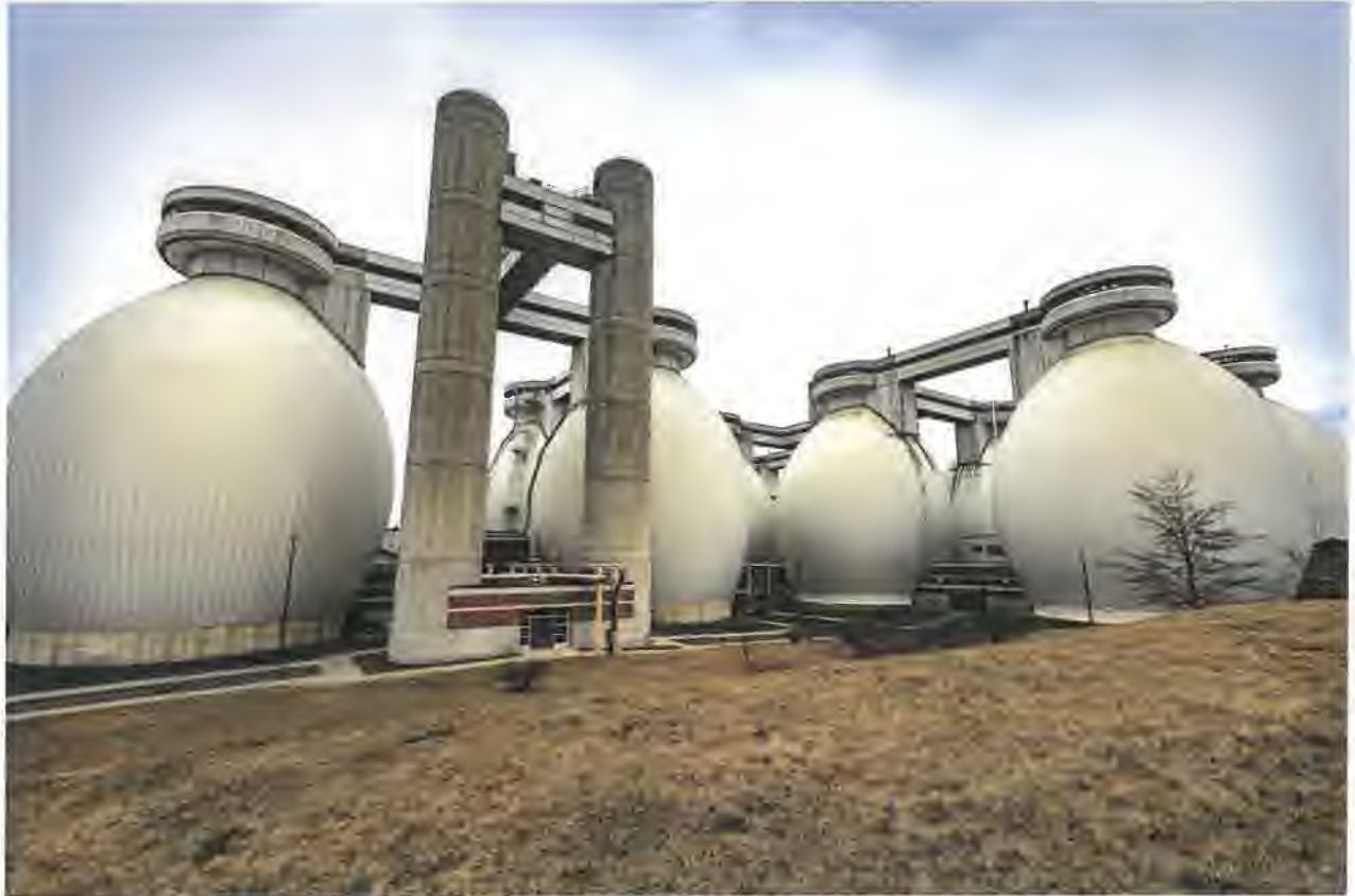
The anaerobic digesters at the Deer Island Water Treatment facility in Winthrop. (Jesse Costa/WBUR)
