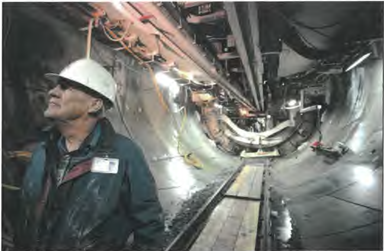
This 1992 photo shows construction manager Joseph Griffith inside the Massachusetts Water Resources Authority's Outfall Tunnel, which would carry sewage more than nine miles underwater from Boston's Deer Island out into the Massachusetts Bay. (Paula Scully/AP)
