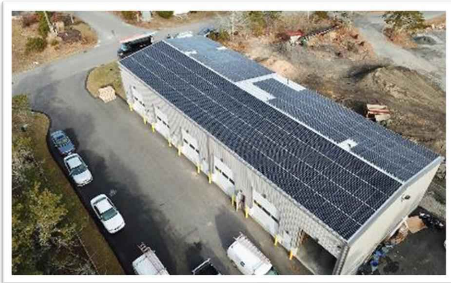
Metal Roof Mounting | 265 solar panels in Chatham, MA Solar Panel Installation by My Generation Energy
