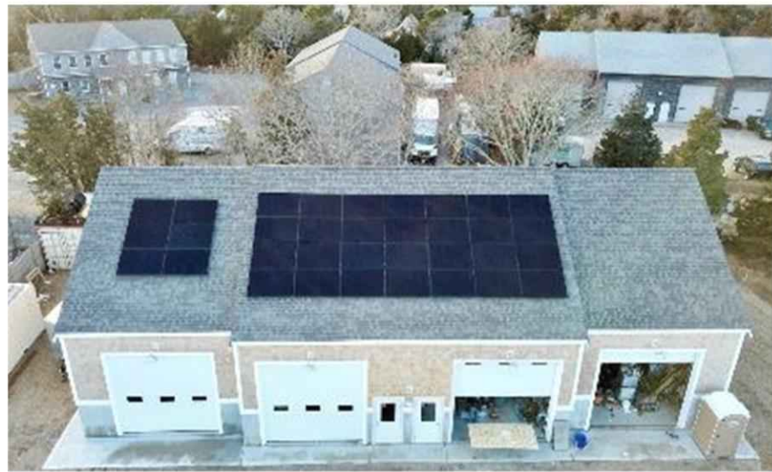
Asphalt Roof Mounting | 34 solar panels in Eastham, MA Solar Panel Installation by My Generation Energy
