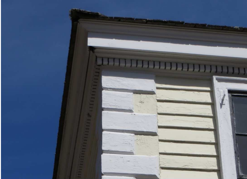
Exhibit F, Photo 3 - Cobb House, detail of cornice and quoining, front elevation, southwest corner.
