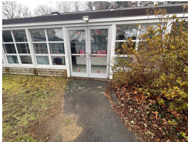
5. Shingles in some areas are too close to finish grade.
