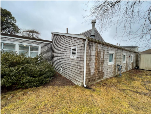
13. Window has failed and lack of adequate overhang at eave has damaged siding.
