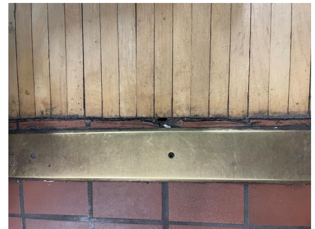
6. Quarry Tile and hardwood floor in Cafetorium are worn.
