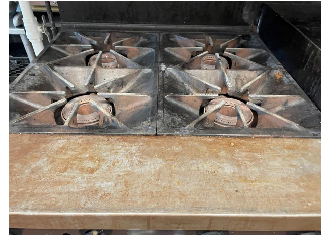
3. Kitchen equipment is outdated.
