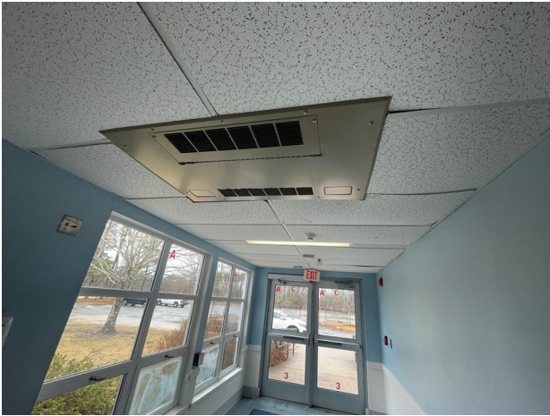
1. Ceiling unit heaters at entry points are outdated.
