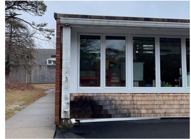
15. Downspout is damaged and water is creating stains on CMU & siding.
