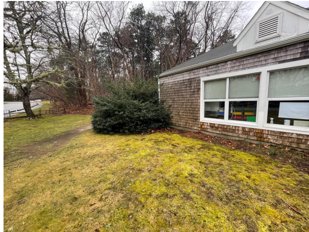
17. Wood trim is damaged.
