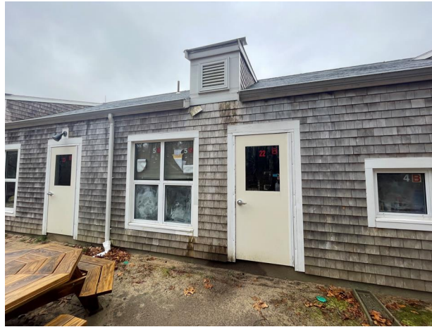
14. Water damage is evident at vent dormers.
