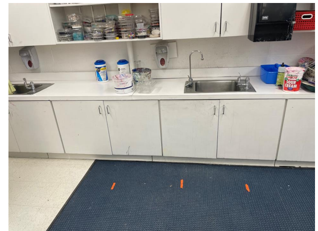
6. Sinks and drinking fountains are not accessible.
