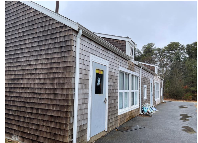
18. Hollow metal door has rust and oxidized paint. Wood fascia is peeling.
