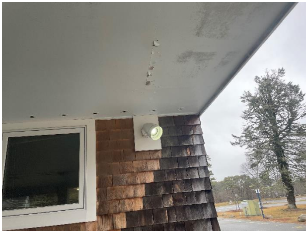
4. Paint is peeling on soffits.
