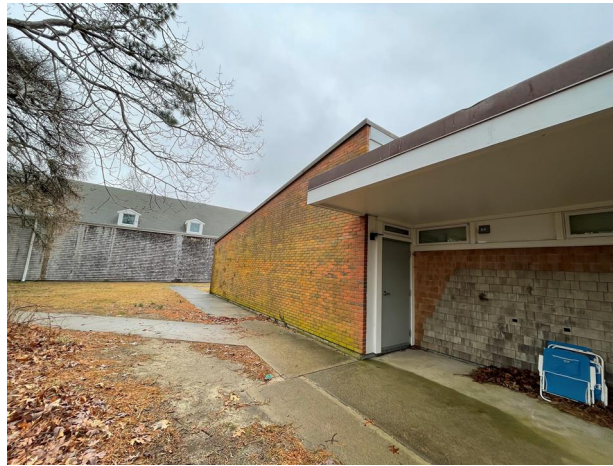
2. Brick is discolored on north elevation.
