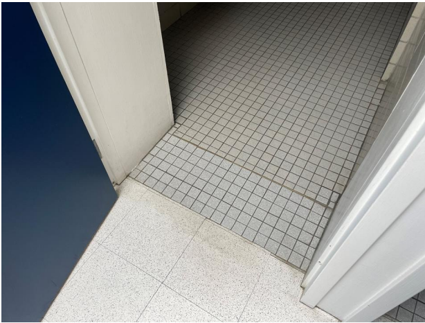
4. Ceramic Tile in Toilet Rooms is damaged.
