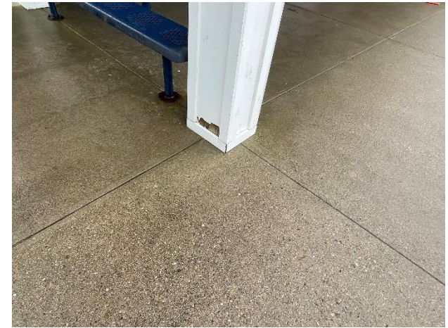
3. Column covers are water damaged.
