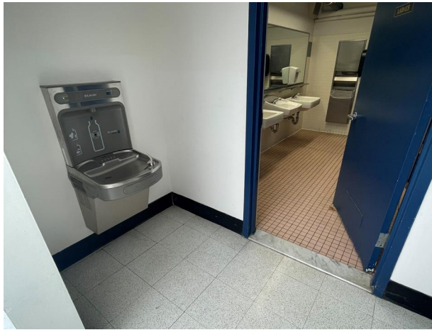
2. There is inadequate clearance at drinking fountains.
