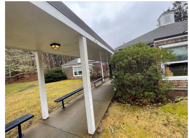
6. Soffits and wood fascia is peeling.
