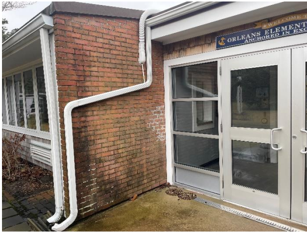
1. Brick is discolored adjacent to main entry.
