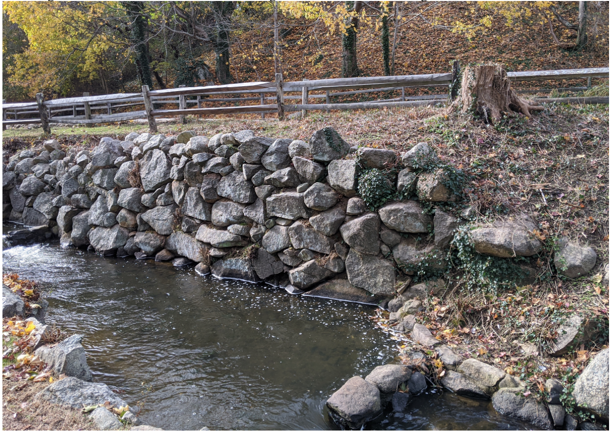
Photo 2. Retaining wall is slumping, rocks at base misplaced, and path above is slumping.
