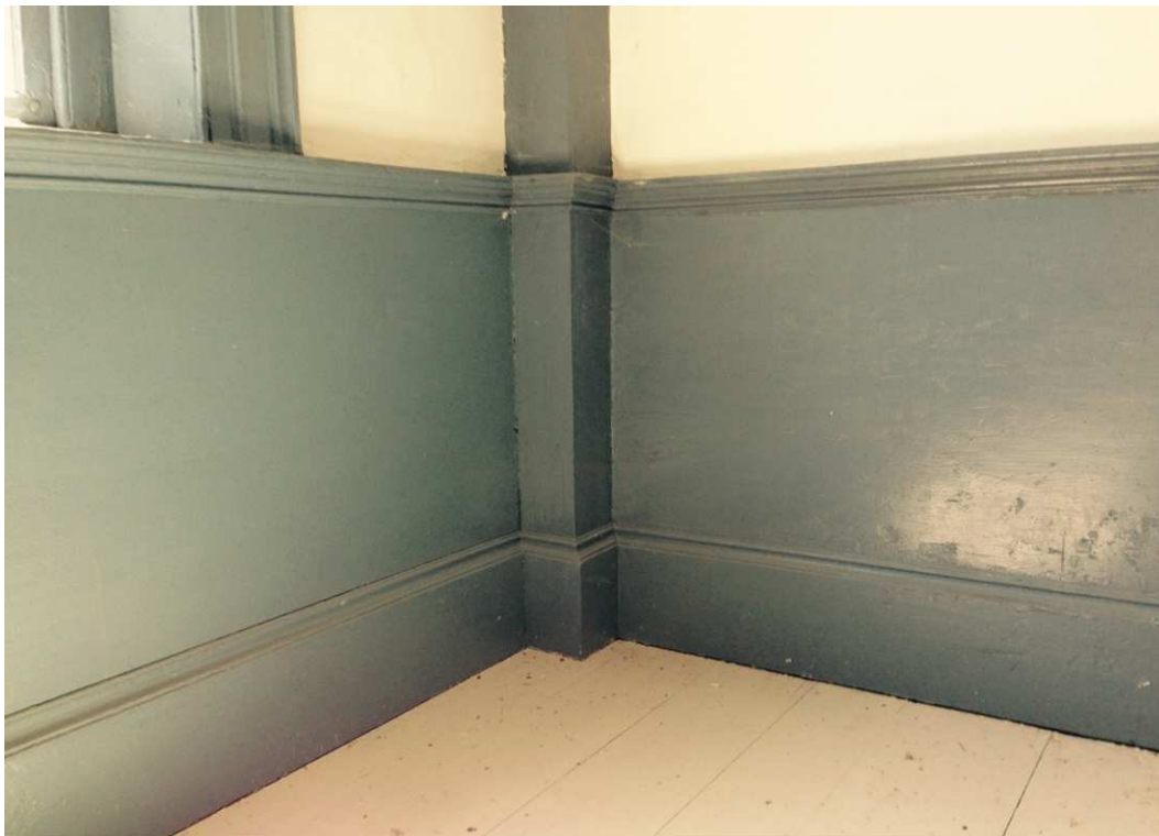
Exhibit F, Photo 33 - Cobb House interior, Southwest Bedroom, detail of wainscoting, southwest corner.
