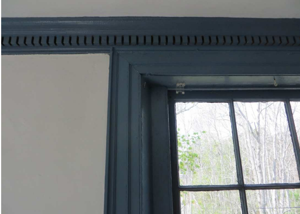
Exhibit F, Photo 35 - Cobb House interior, Southwest Bedroom, cornice and window detail.
