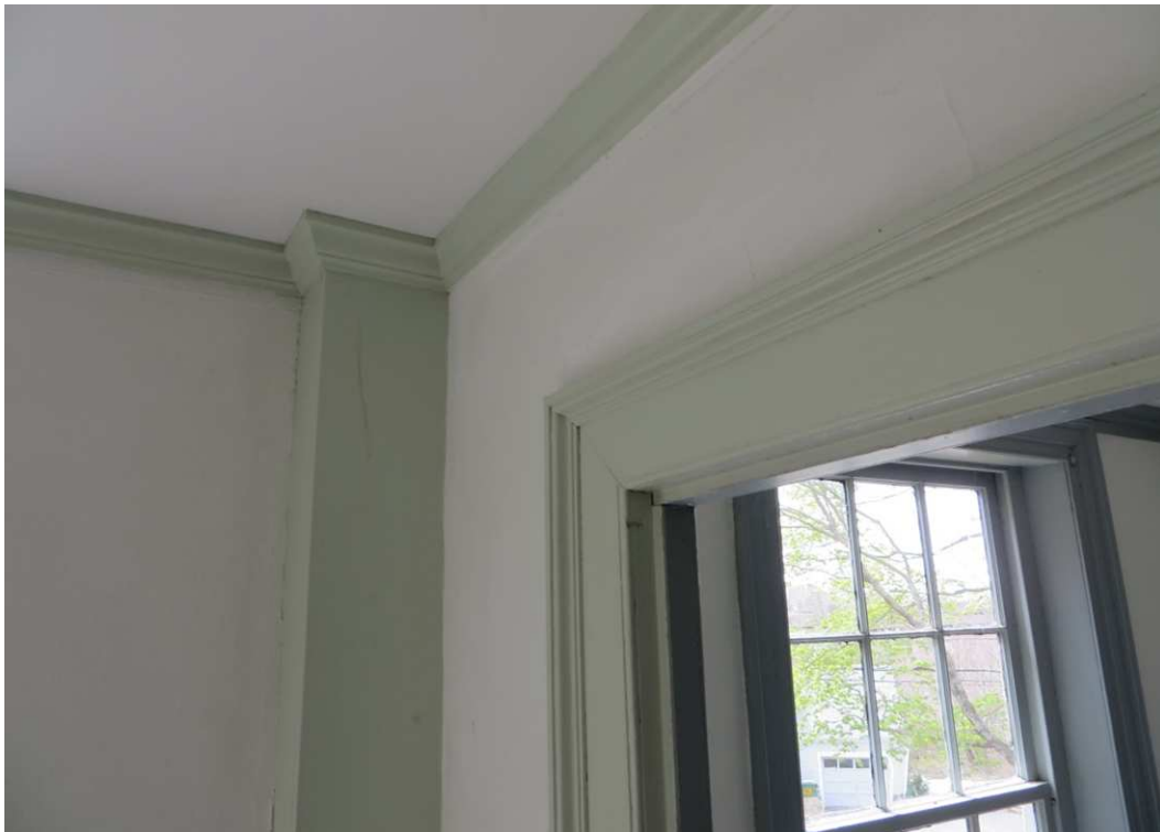
Exhibit F, Photo 42 - Cobb House interior, Southeast Bedroom, detail of door surround, post, cornice.
