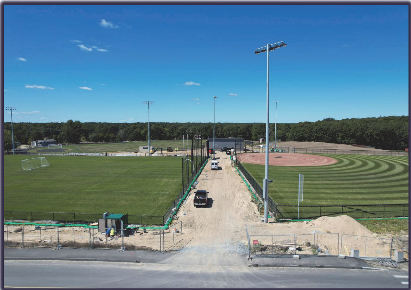
Two new athletic fields are in progress as additions to the existing sports complex.
